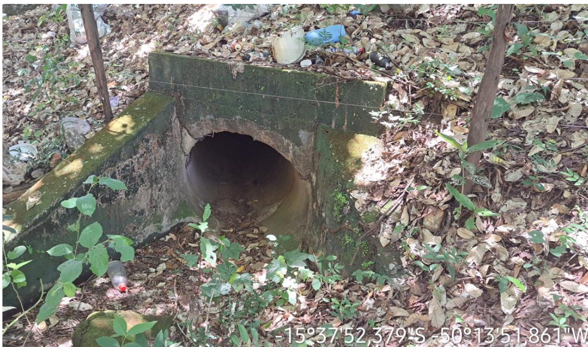
-15^{\circ}37'52,379''S -50^{\circ}13'51,861''W Km: 43,40 – Bueiro tubular.
